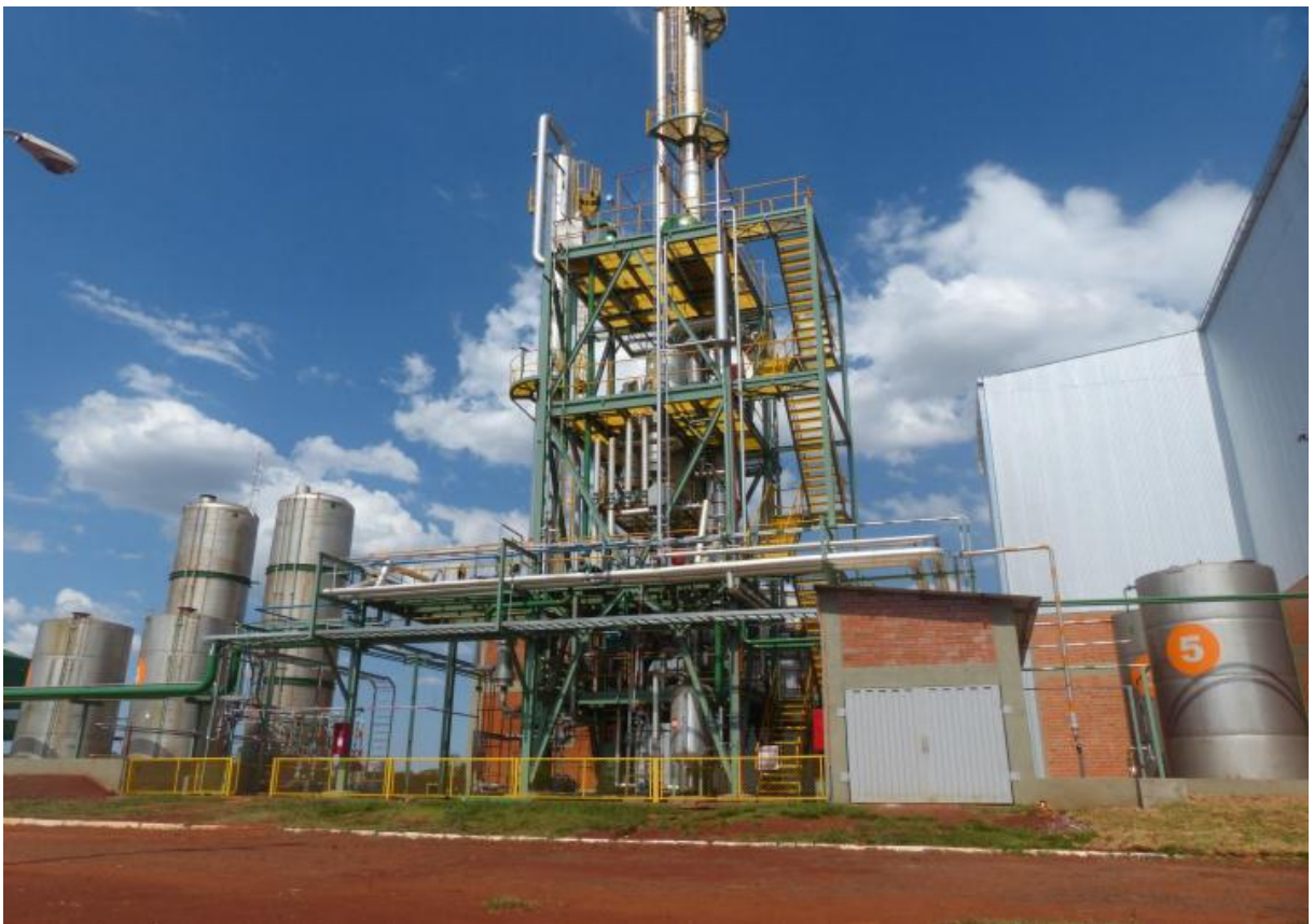
Minga Guazú plant, vacuum tower and topping
