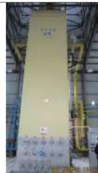
Air separation column
