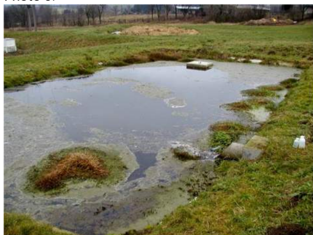
Photo 6: Small Settling Tank Overgrown with Filamentous Algae
