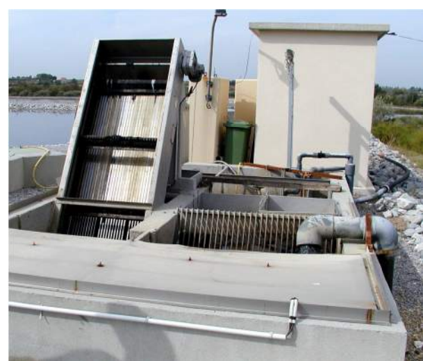
Photo 3a,b: Mechanically Raked Screens
