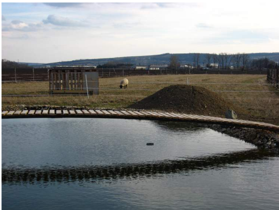
Photo 35: Example of Implementation of Final Treating Biological Tank on the Farm
