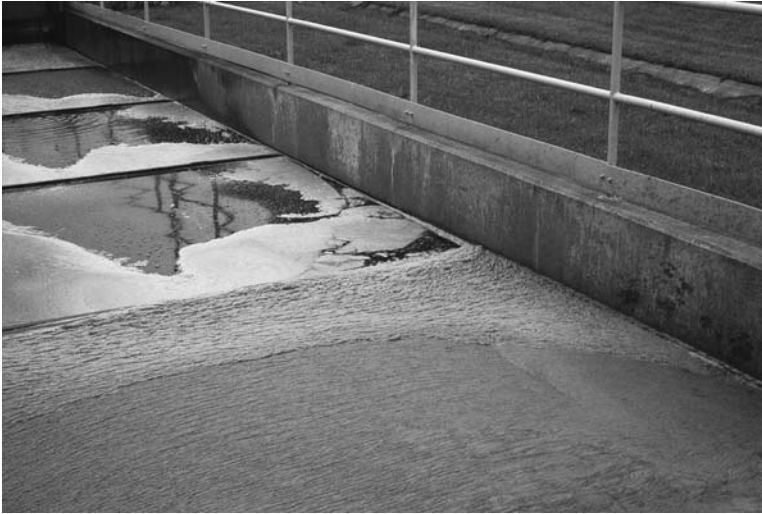
FIGURE 20.2 Collapsed foam or “scum” on the surface of a secondary clarifier.
