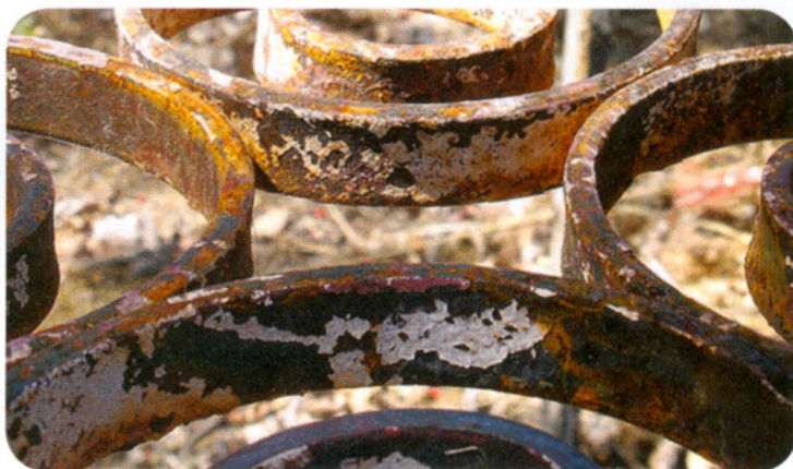
Rusted steel parts.
