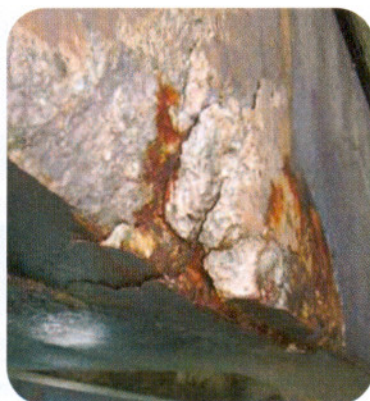
Concrete damage from corroded rebar by salt in marine atmosphere.
