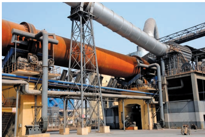
Figure 6.23 Rotary kiln from the cement industry.
