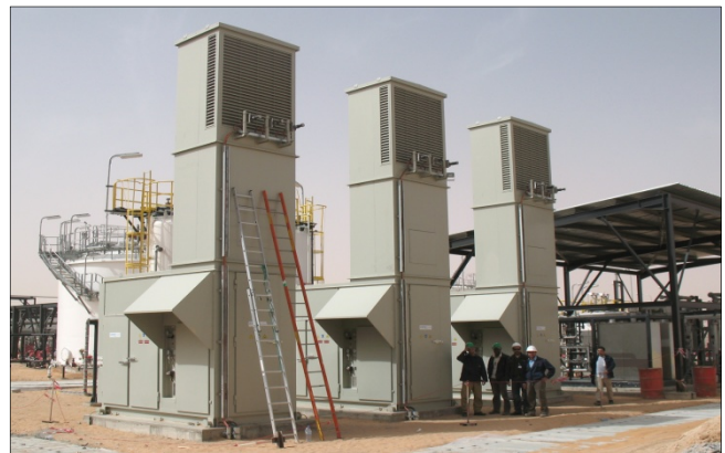
A set of three units on location in Algeria (picture taken during operator training in 2011) each unit with a 160 kW E-motor driven oil-free 2-stage screw.
