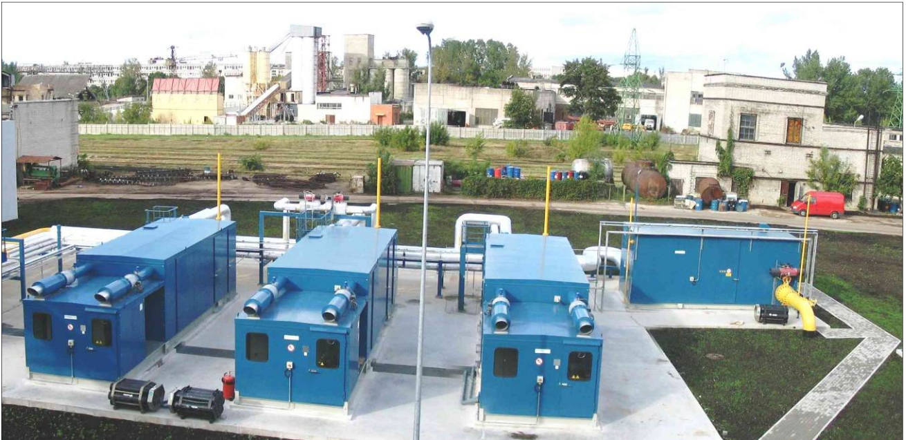
Three identical Eltacon fuel gas booster compressors in Riga – Latvia.
