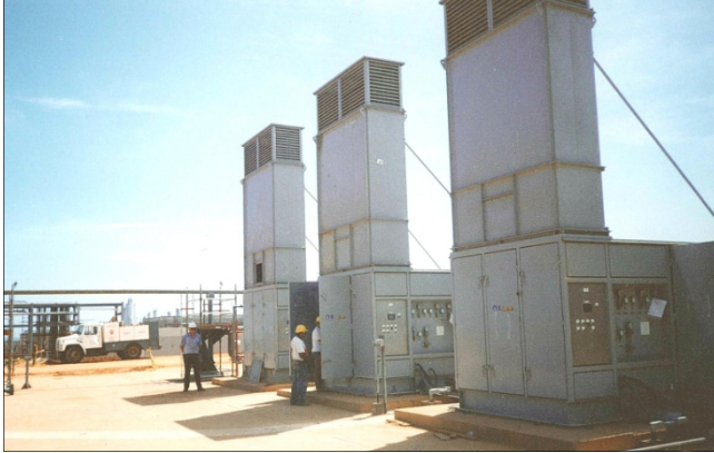
Three oil-free compressors on a site in Venezuela. Two units with a 350 kW E-motor & one unit with a 325 kW steam turbine. In operation since 1998.
