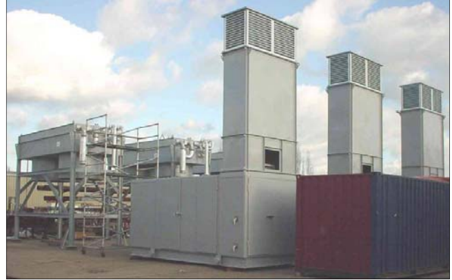
Three air compressor packages during testing. Each package includes a 2-stage oil-free screw that is driven by a 5,5 kV / 510 kW E-motor.
