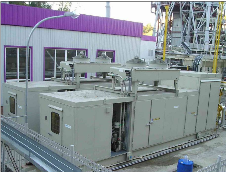
Two identical Eltacon fuel gas booster compressors in Sochi – Russia, each with an oil-lubricated screw driven by a 3 kV, 650 kW E-motor. Gas is being compressed from 9 barg up to 27 barg. Capacity 2x 7.763 kg/h.
