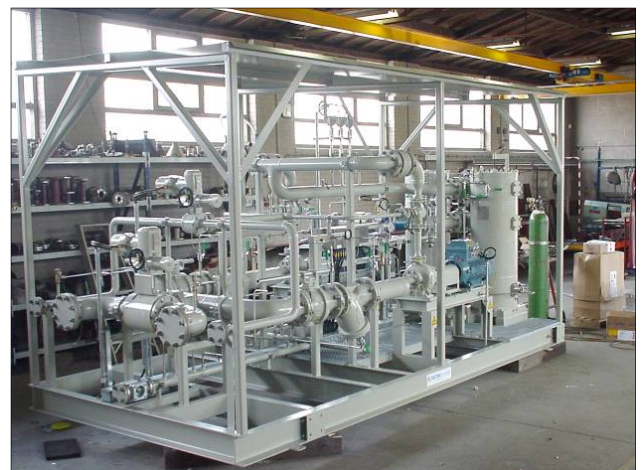
At the right a liquid fuel system, with two (100%) oil conditioning lines each with fuel pump, coalescing filters, valves, controls etc. for liquid-fuel firing of dual-fuel gas turbines.
